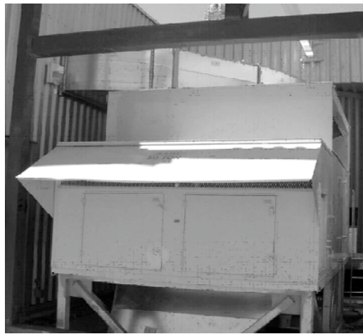
FIGURE 2 DATA CENTER CONVERTED TO USE AN AIRSIDE ECONOMIZER
